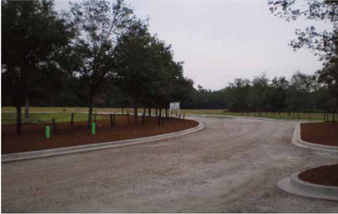
Road work continues at The Settings of Mackay Point. The curbs are in at the Front Entrance.
