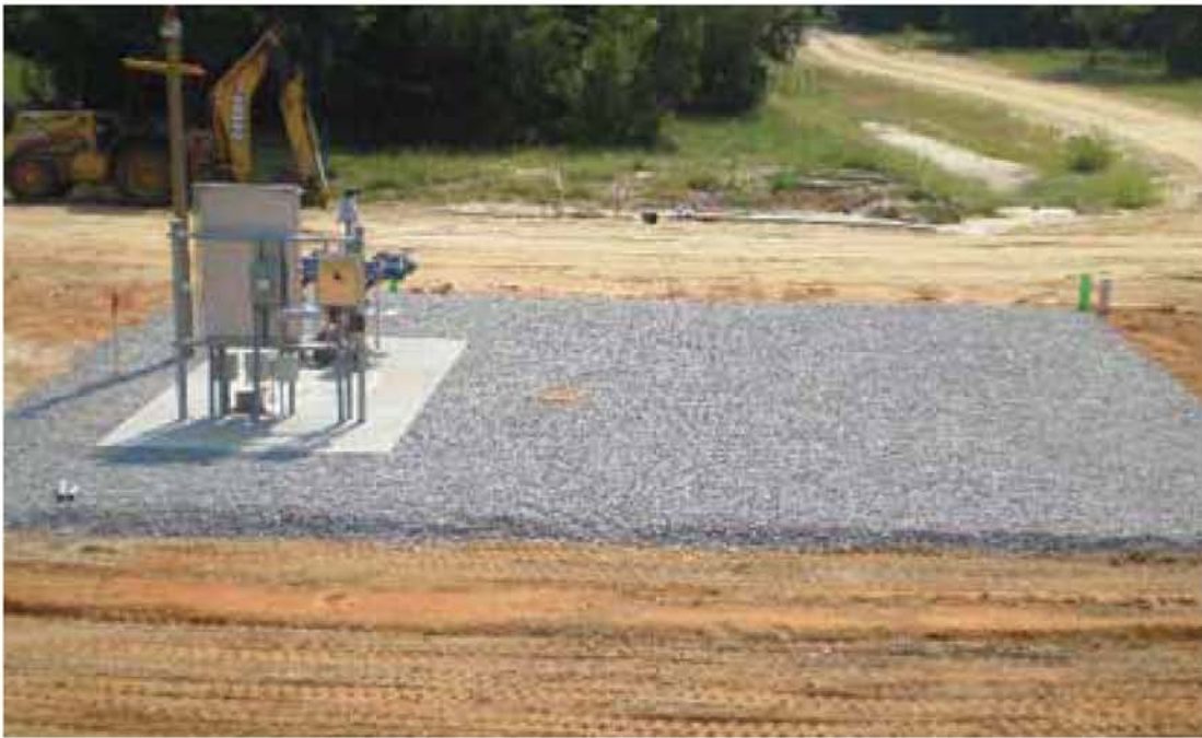
2 pumpstations are installed. 1 will serve phase 2 West and 1 will serve Phase 1 and Phase 2 East.
